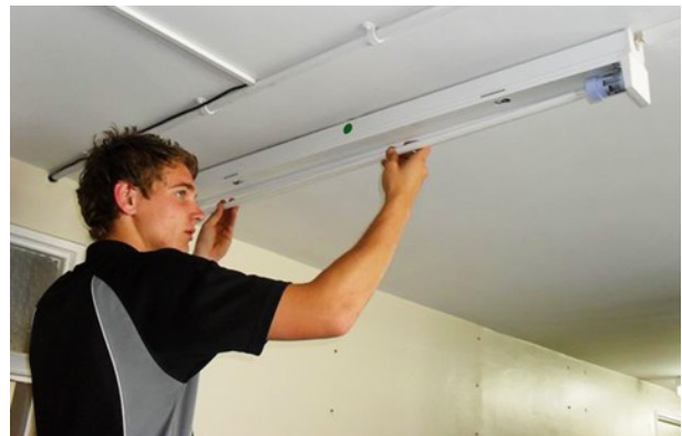
Jacob Manaton from Mark Woofe Electrical shows just how easy it is to install ecoBright® T5 adaptors - this upgrade was completed quickly and efficiently due to the professionalism shown by the installers...thanks guys!
