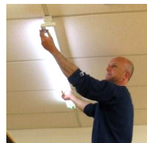
SKY's Electrician Danny Courtenay completes retro-fitting a double lamped T8 luminaire with T5 lamps using Save It Easy® at SKY offices in Mt Wellington Auckland.
